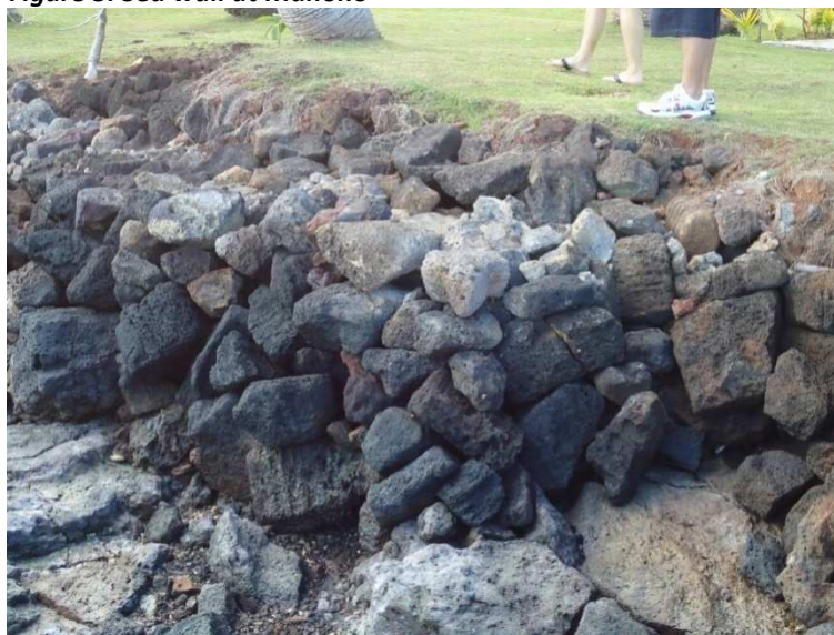
Figure 5. Sea wall at Manono
